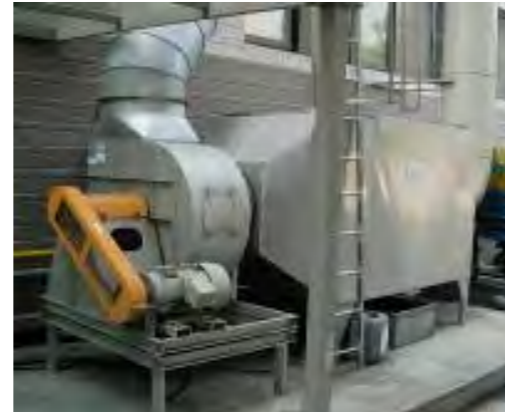
Activated carbon adsorption tower
